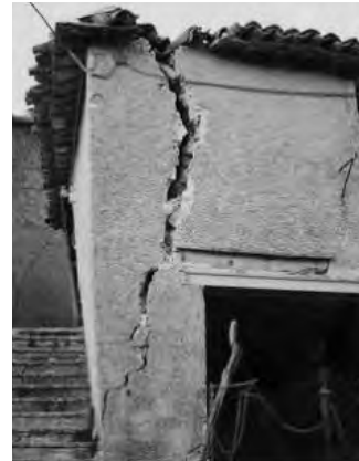
Figure 4. In this masonry building it is possible to see the overturning of the wall caused by a poor connection of the roof to the wall.
