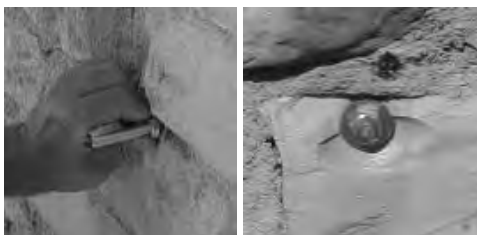
Figure 8. Positioning of stainless steel threaded bars used as ties: a) fixing of the nut; b) external aspect of the strengthened wall.
