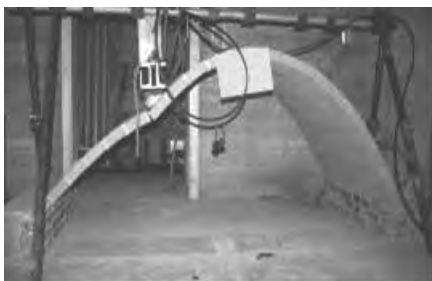
Figure 14. Collapse mechanism of a vault strengthened using CFRP strips (Valluzzi et al., 2001).
