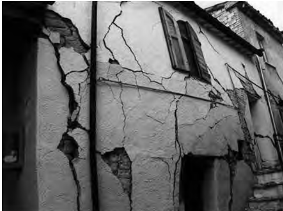
Figure 3. In this masonry building it is possible to see a flexural wall failure. There is a good roof-to-wall connection but the middle floor is not connected to the wall. In this case we can see how important is to achieve the connection between the roof and the existing masonry.
