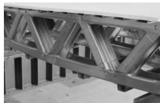
Figure 18. Collapse due to combined shear-tensile failure of rivets.
