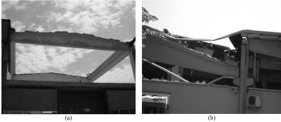
Figure 4. Roof elements collapse due to the loss of support from main beam (a) and loss of support of beam from column (b).
