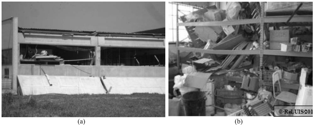
Figure 5. Collapse of horizontal precast panels (a) and damage to storage racks (b) with consequent loss of contents, as surveyed in a number of industrial buildings.
