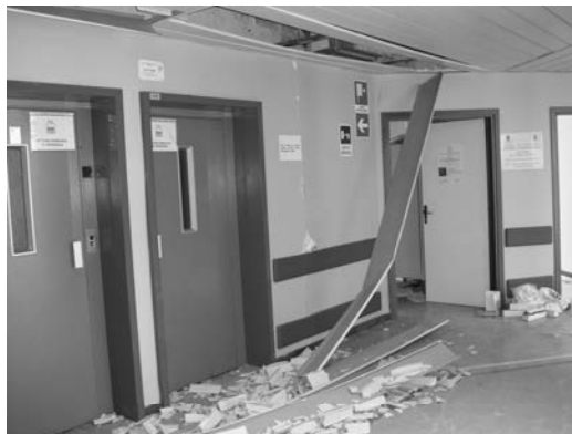
Figure 1. Hospital “San Salvatore dell’Aquila”: ceilings failure.
