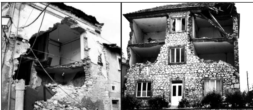
Figure 12. Tilting of the wall along shear-lesions diagonal direction.
